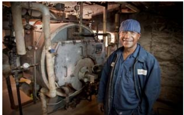
James Miner, a maintenance worker at the Morrisiana building, stands alongside a boiler he monitors each heating season.
